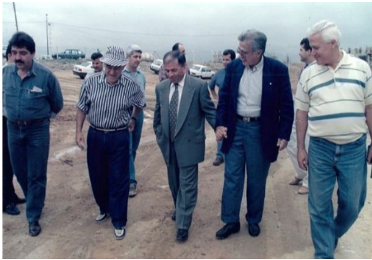
Photo 6. Professor Mehmet Hıfzı Özcan and Sakip Sabanci, at the Metin Sabanci Center construction site
