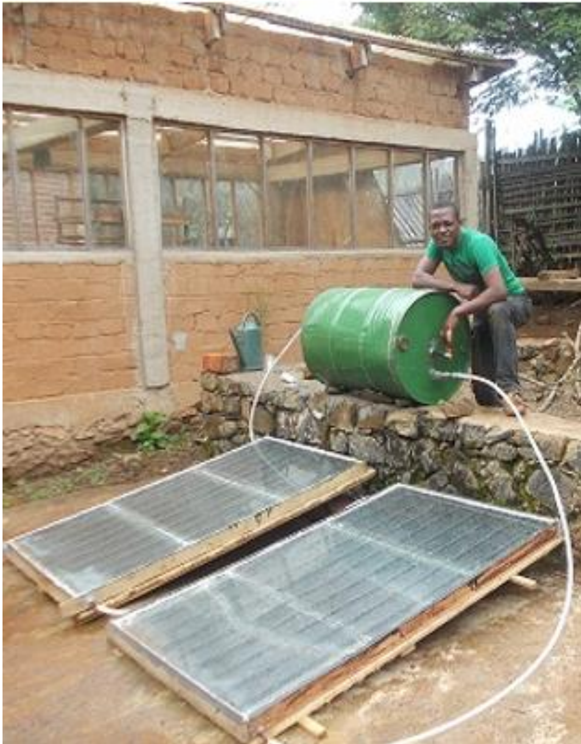
Figure 7. Final TSWH system designed, manufactured and installed.
