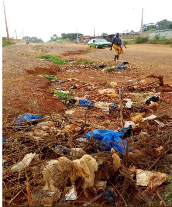
Figure 8. Degradation of an unpaved road in the South D district
